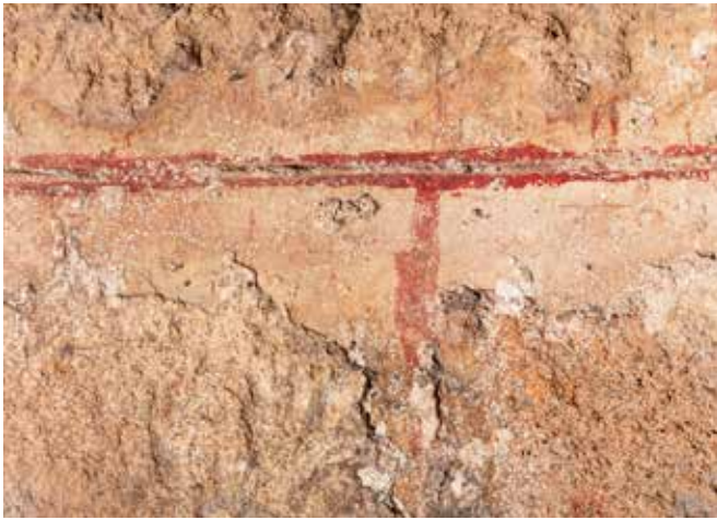
15 Space between Torre Pisana and Joharia, external masonry of the Torre Pisana, with engraved and red painted grooves over the joints between the blocks (Palermo, Palazzo Reale)
