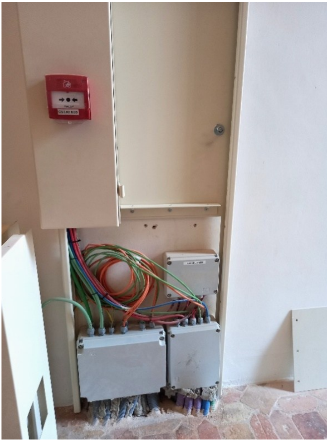
129 Detail of the totem containing electrical systems, 2024 (A. Fapanni)
