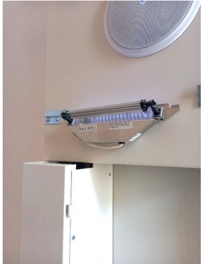
130 Detail of the totem containing electrical systems, UV insect trap, 2024 (A. Fapanni)
