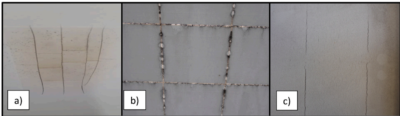
Fig. 20. Common failures in PV backsheet due to thermo-mechanical and material degradation: (a) cracked backsheet beneath a hot Si-cell, (b) squared cracks beneath cell interspaces, and (c) longitudinal cracks located beneath bus-bars, from Eder et al. (2019).
