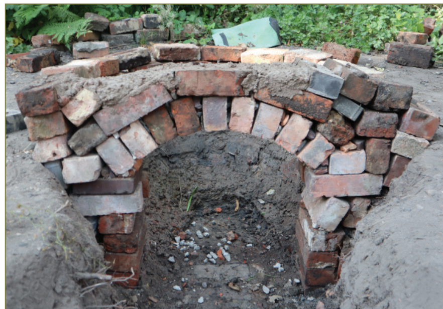
Fig 6 (Below). Building the arch with a wooden arch-shaped frame. Photo by Tomei and Jiménez Rivero.
